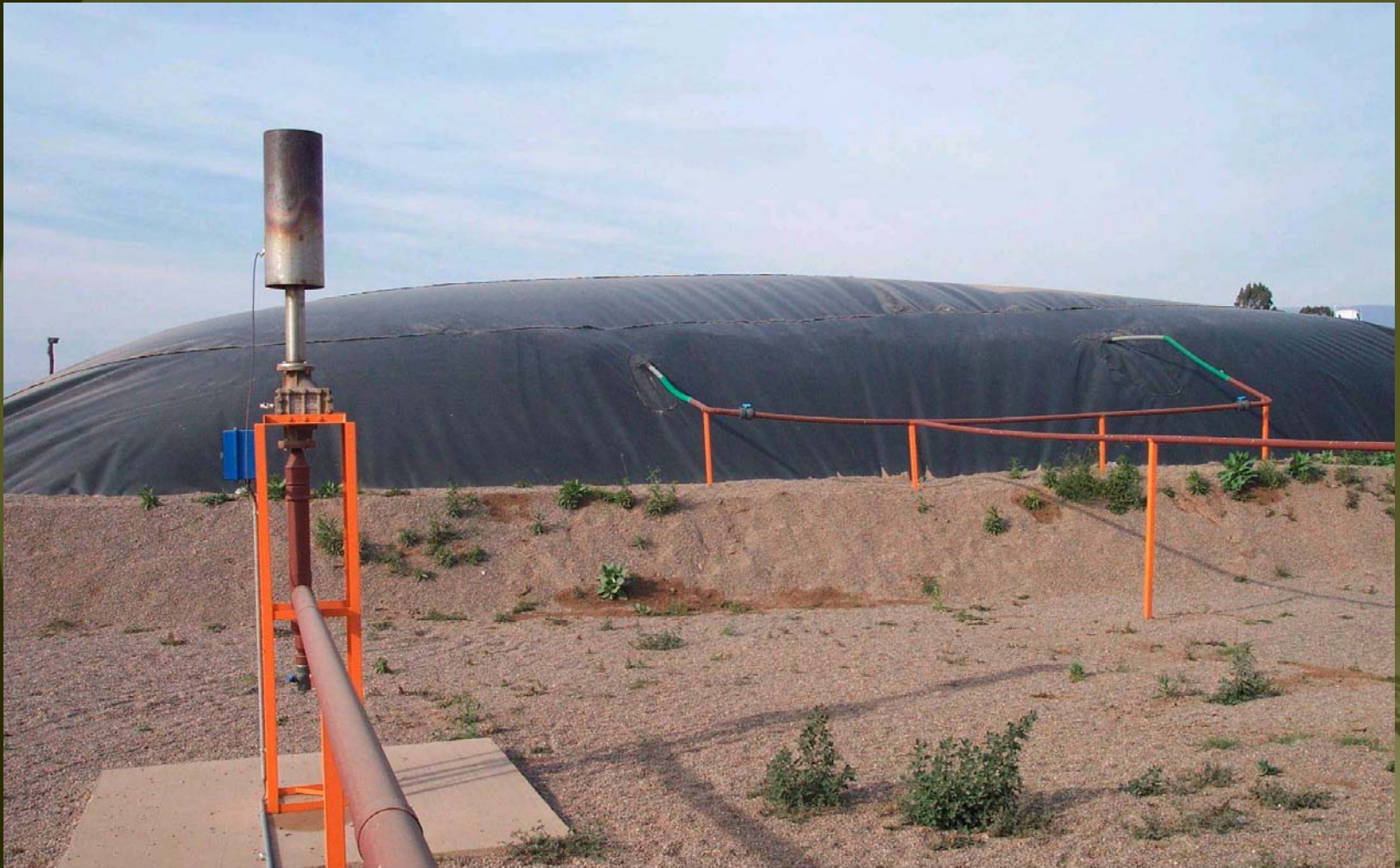
Photo 1 - Energy Cell, Landfill Gas Pipes and Flare
