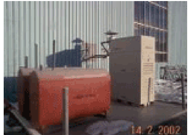
Microturbine, Tufts Cove NS
