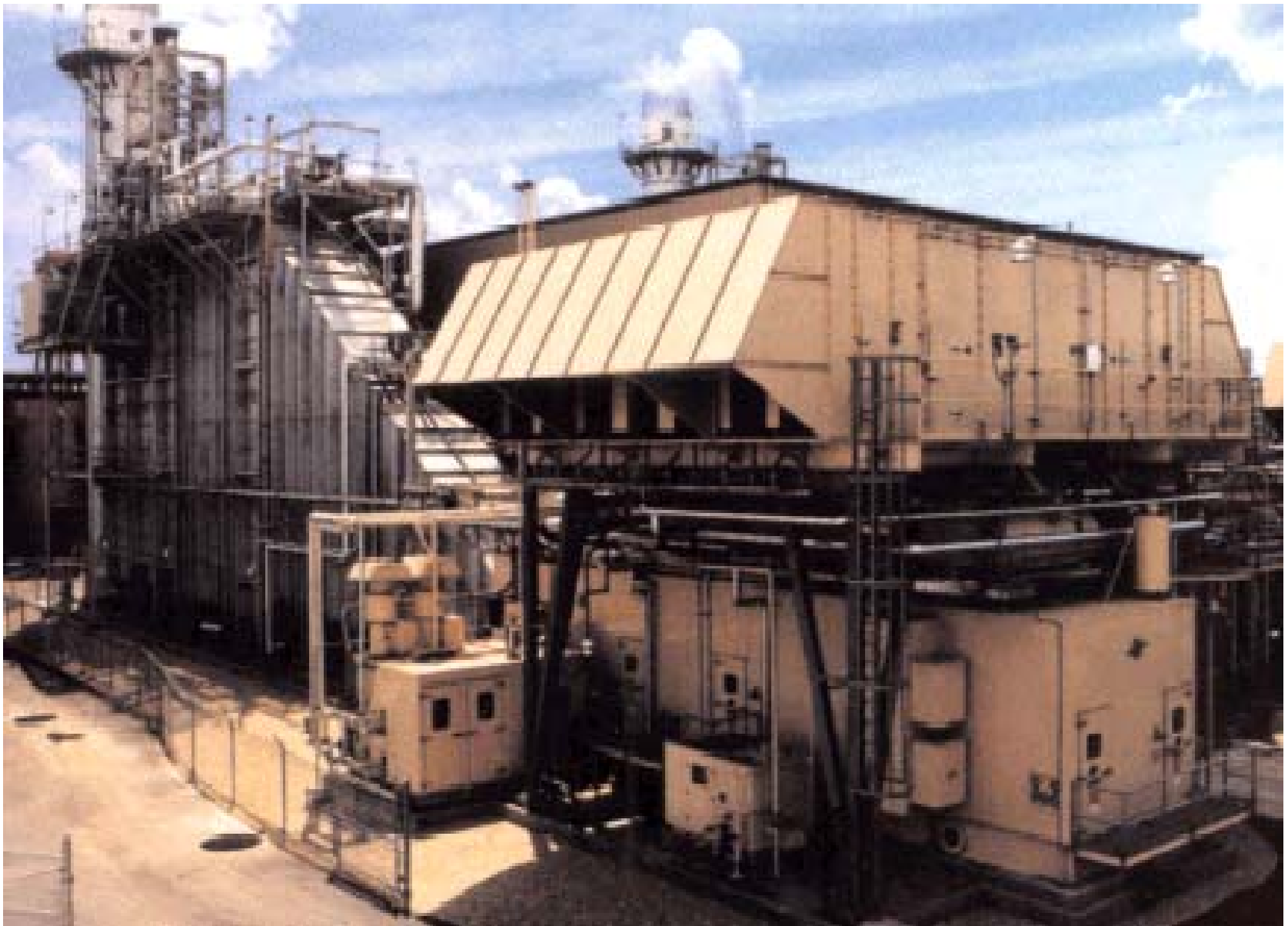
Gas Turbine & Heat Recovery Steam Generator (GE Power Systems)
