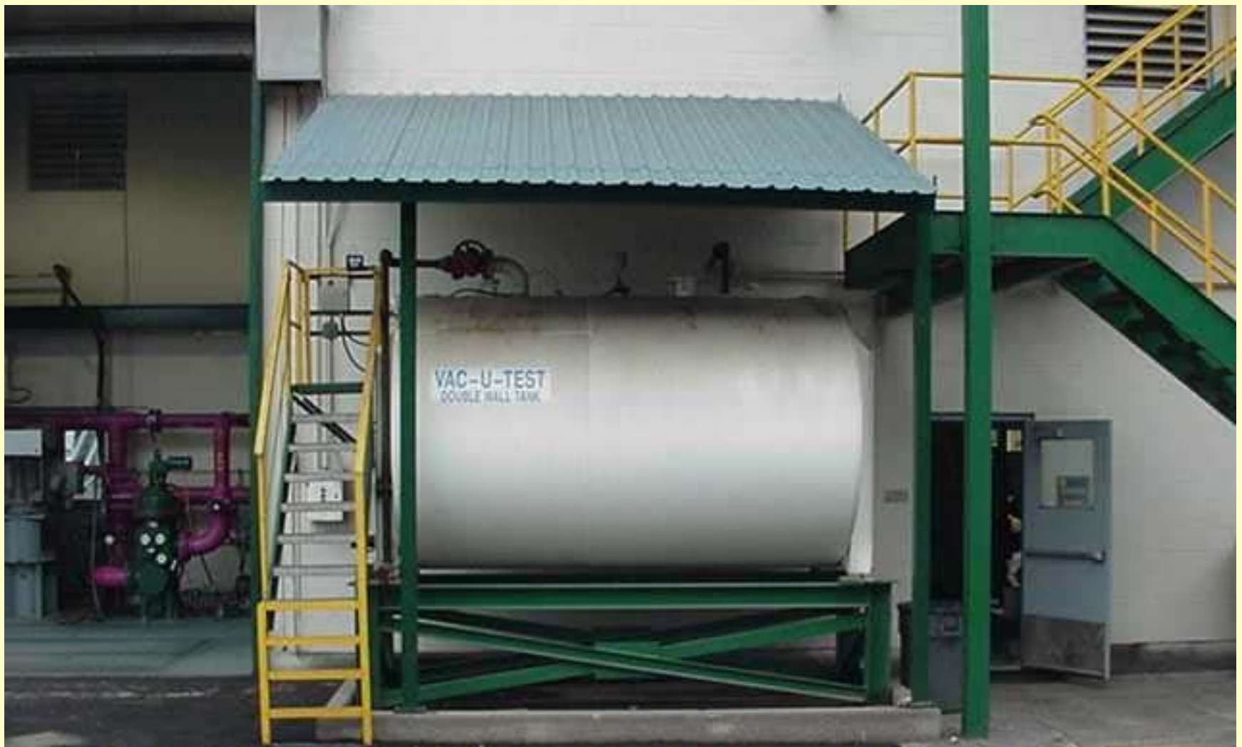
Hydraulic Oil Tank with roof and secondary containment
